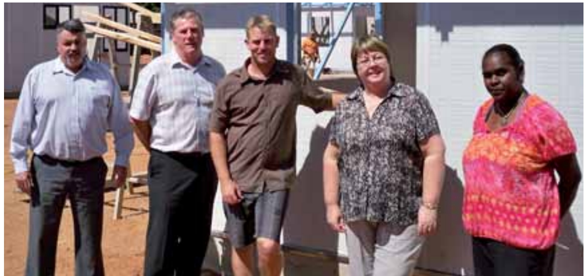
Napranum Council CEO Margaret Barnes (second, right) and the council's housing officer Lima Boseun joined QBuild's Rick Parmenter and Alex Walsh and project manager Philip Gerchow to inspect a new home.
